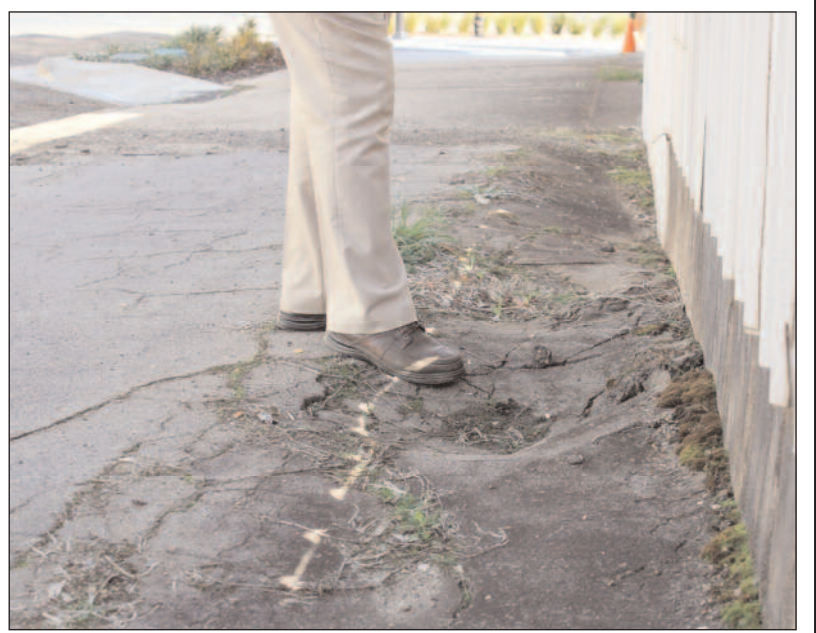
Footpaths in Gundagai will see renewal and repairs when Council undertakes its footpath renewal and replacement Stronger Communities Fund major project.
